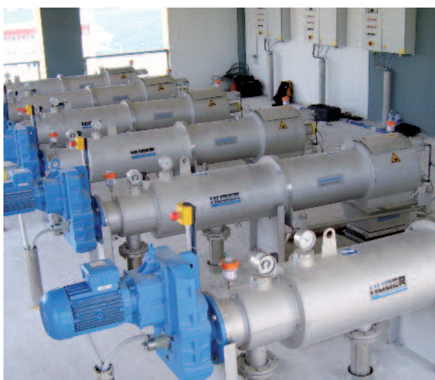
Sludge screening on WWTP Barcelona, Spain
