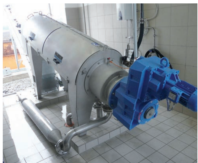
Stationary unit dewatering 140 kgDR/h
