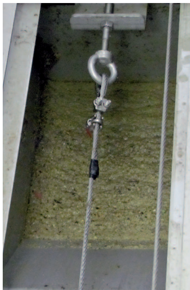
Paddle scraper for grease removal from the grease trap. According to the principle of a longitudinal grit removal scraper the grease paddle pushes the floating fat and grease into the pump sump.
