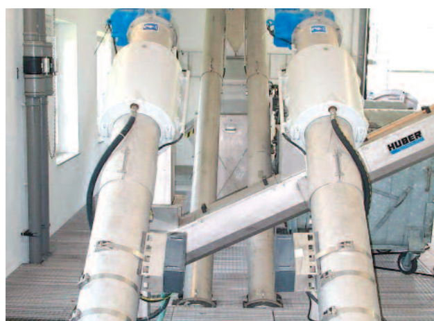
Underground, redundant ROTAMAT® Complete Plant Ro5
