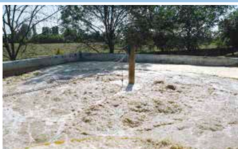
Aeratori sommersi tipo SC installati in impianto di depurazione. Submersible aerators type SC installed in a wastewater treatment plant.
