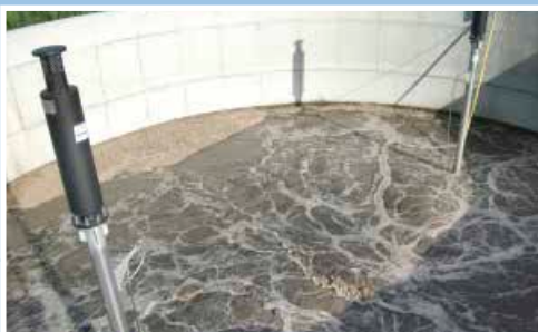
Aeratori sommersi tipo SC installati in impianto di depurazione. Submersible aerators type SC installed in a wastewater treatment plant.
